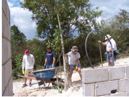
Kyle, Briane, Jeanette and Tony shovel sand into the Habitat house for the floor.
